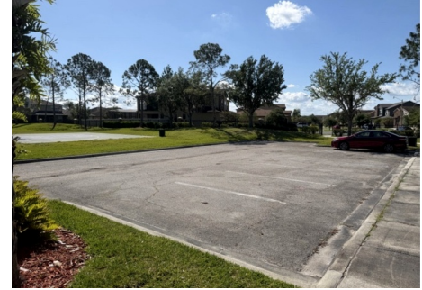
Existing pavement wear
