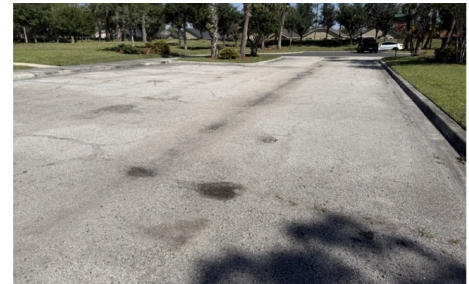
Surface staining / ponding
