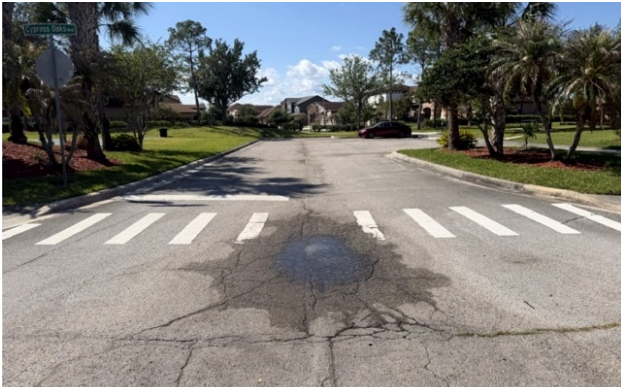
Existing Cracking & Surface Wear
