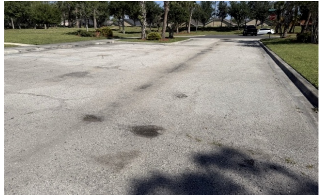
Oxidation & Ponding Evidence
